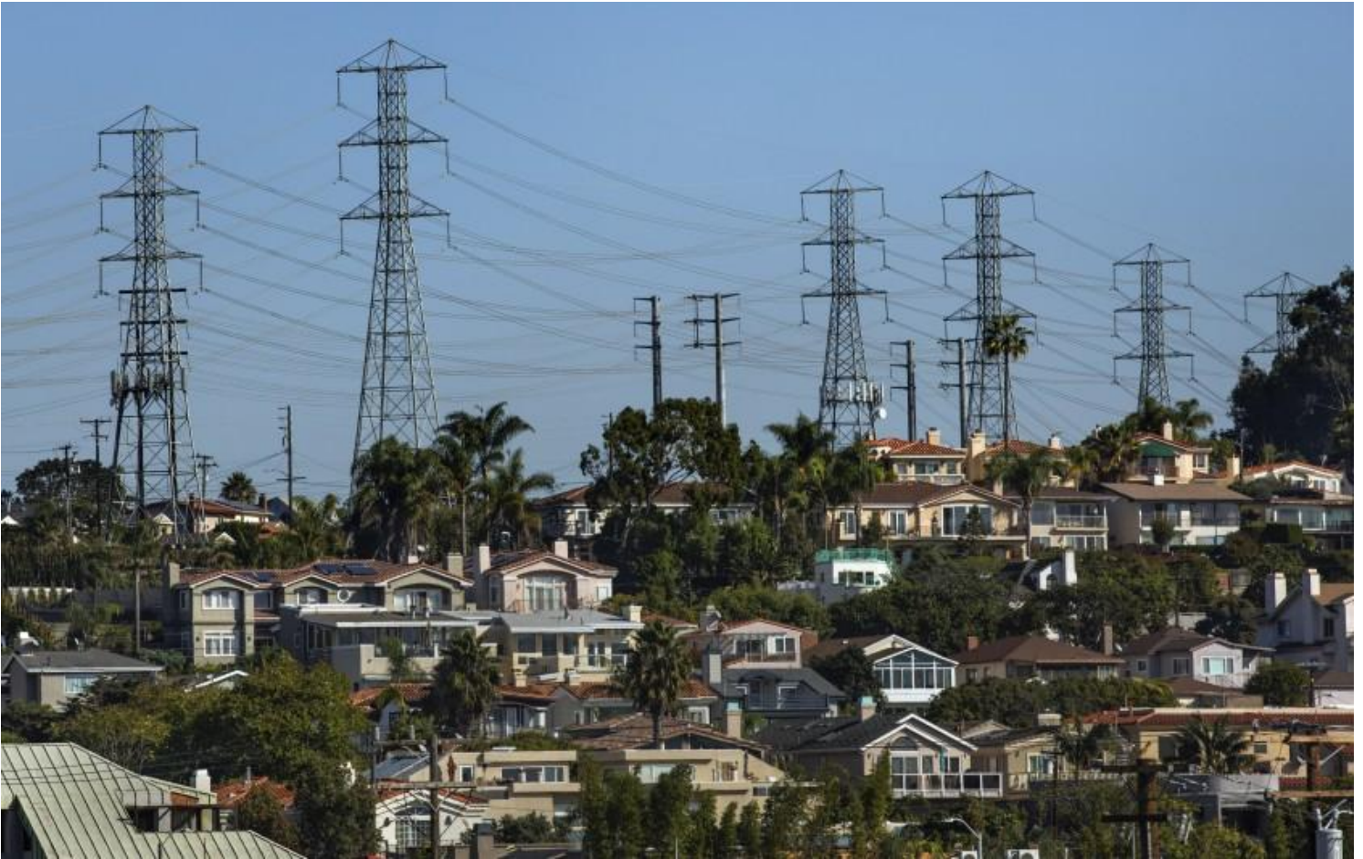
Power lines carry electricity from the AES gas-fired plant in Redondo Beach toward a substation several miles inland, by the 405 Freeway. (Mel Melcon / Los Angeles Times)
